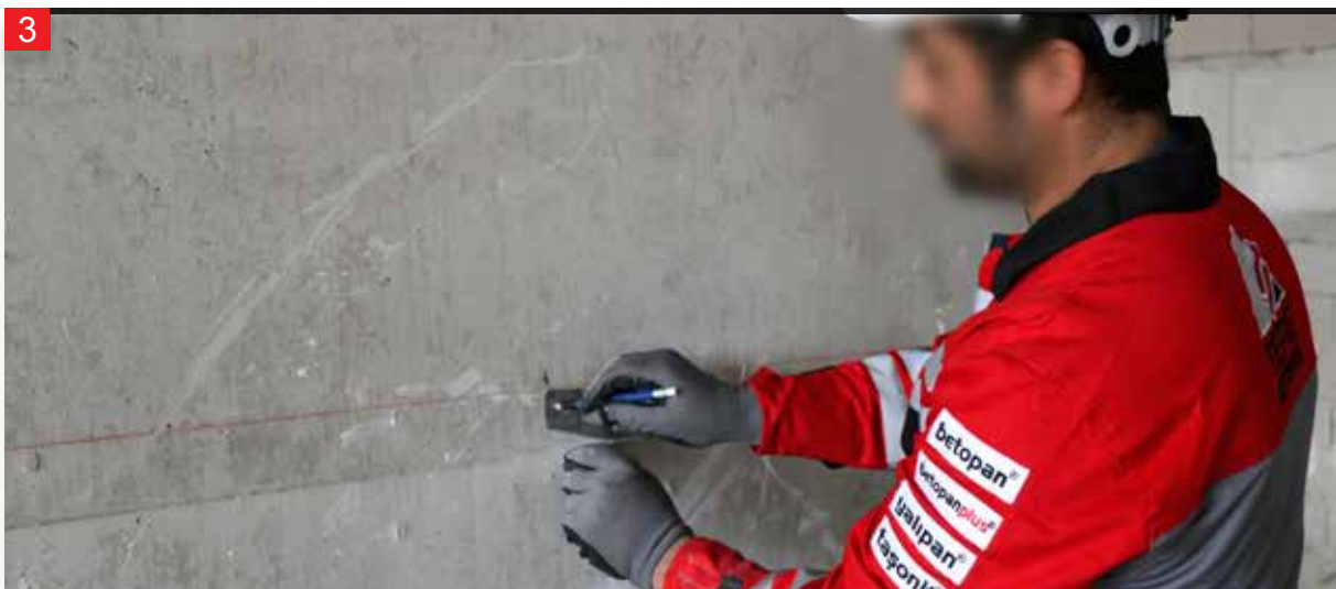
The places to drill for fixing the L consoles to the wall with dowels are marked.
