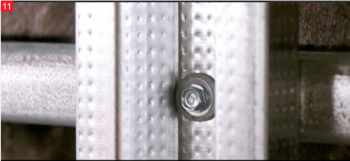
The M profiles are attached to the surfaces of L profiles, for which the leveling has been checked, using triphone self tapping screws screwed on to the center of the L profiles as shown in the photograph.
