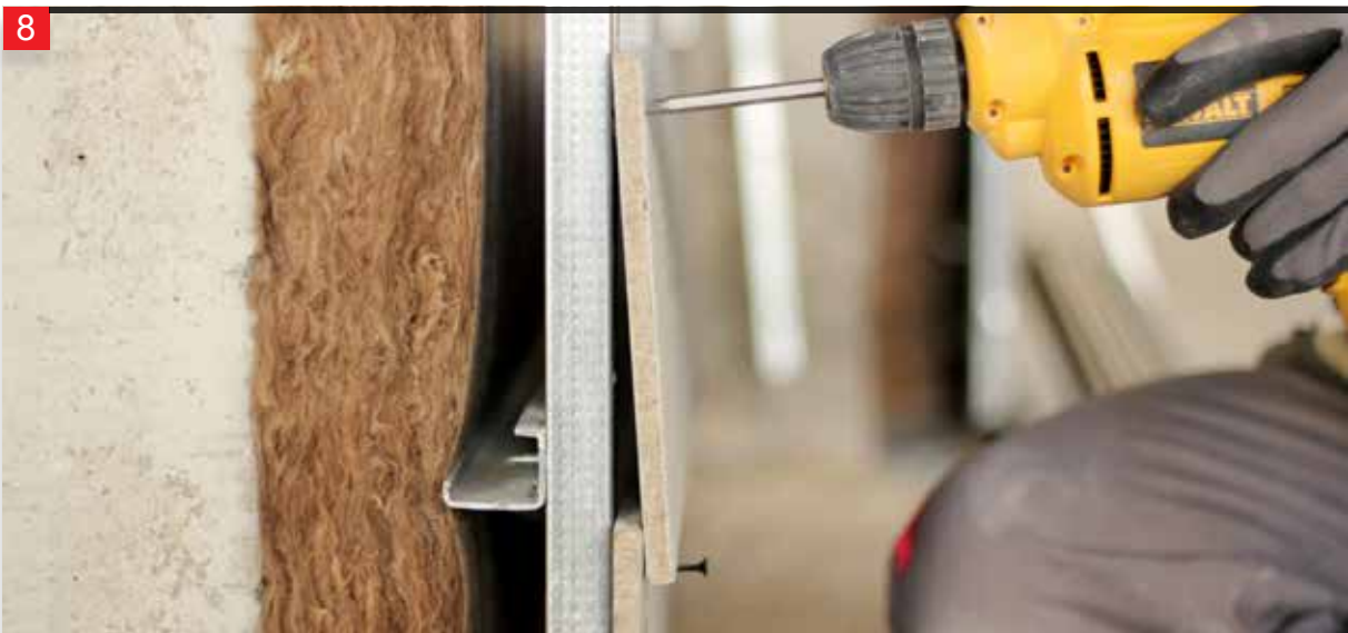
The subsequent overlapping panels are aligned and screwed on the M profile surface.
